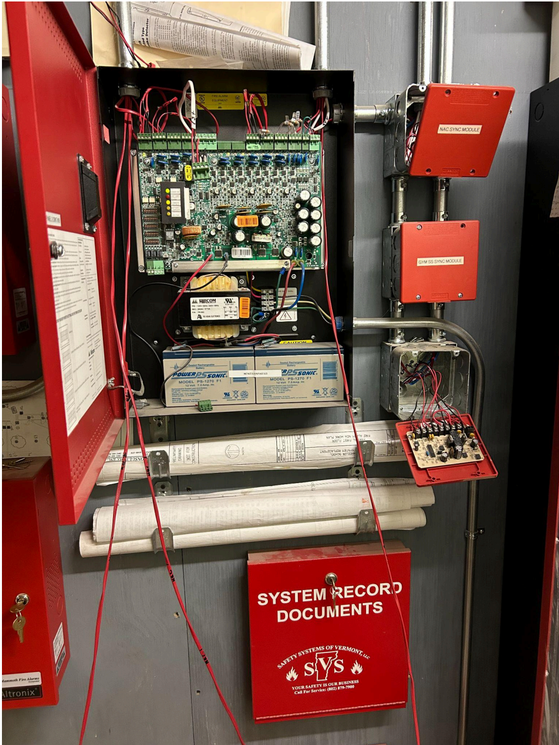
Fire Alarm subpanels
