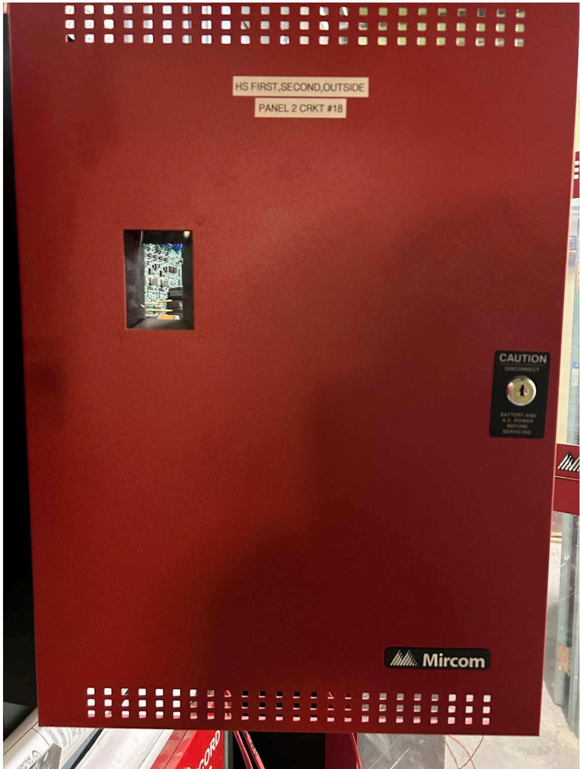
Picture of door of the subpanel above.
