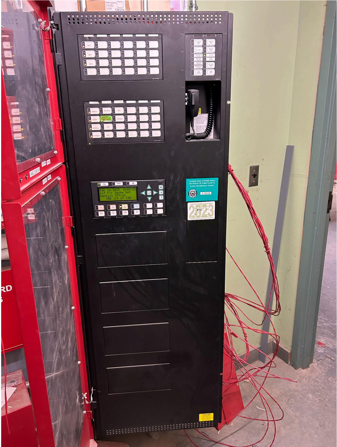
Main Fire Alarm Panel
