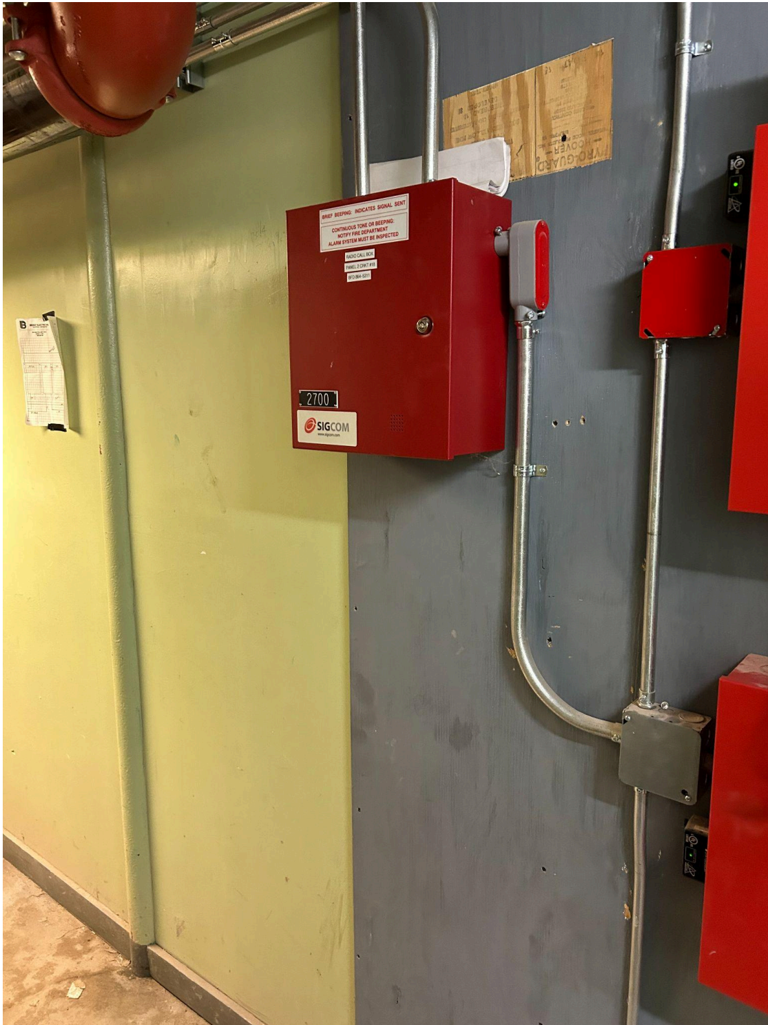
Last of the Fire Alarm subpanels.
