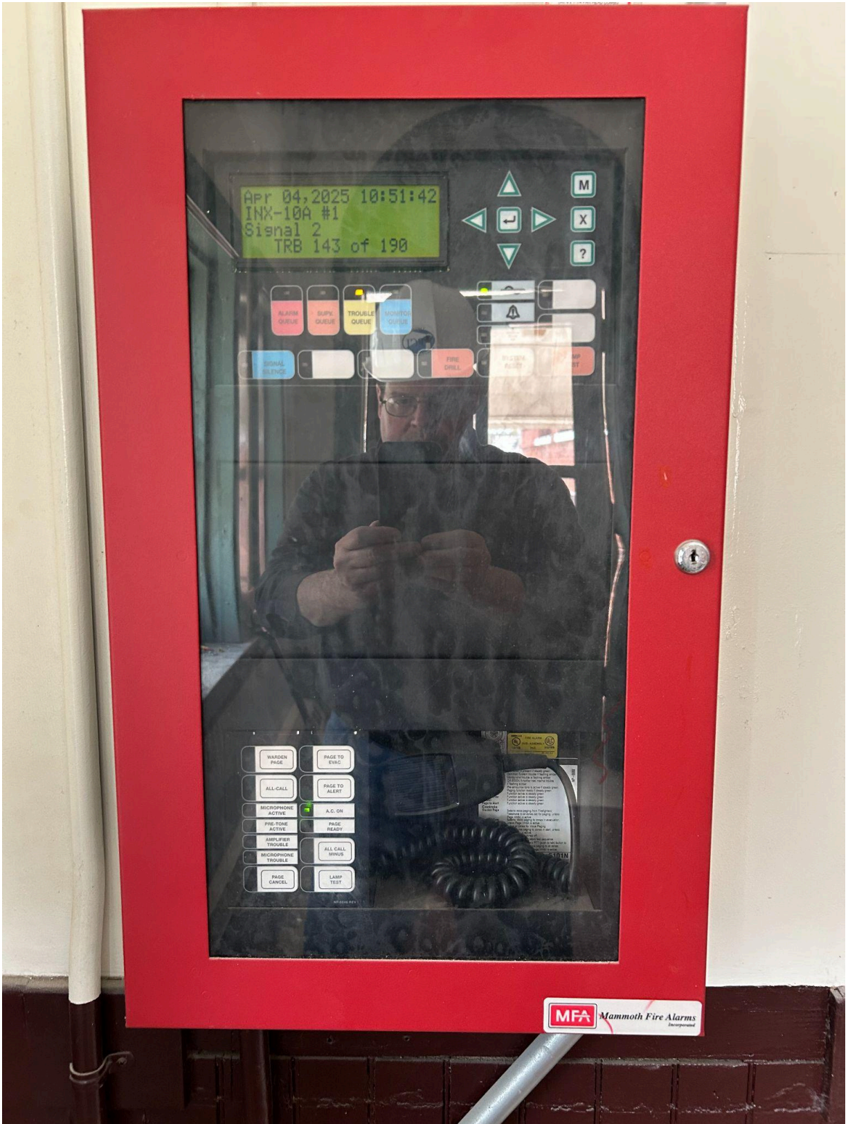
Picture of the Fire Alarm Subpanel in the stairway.
