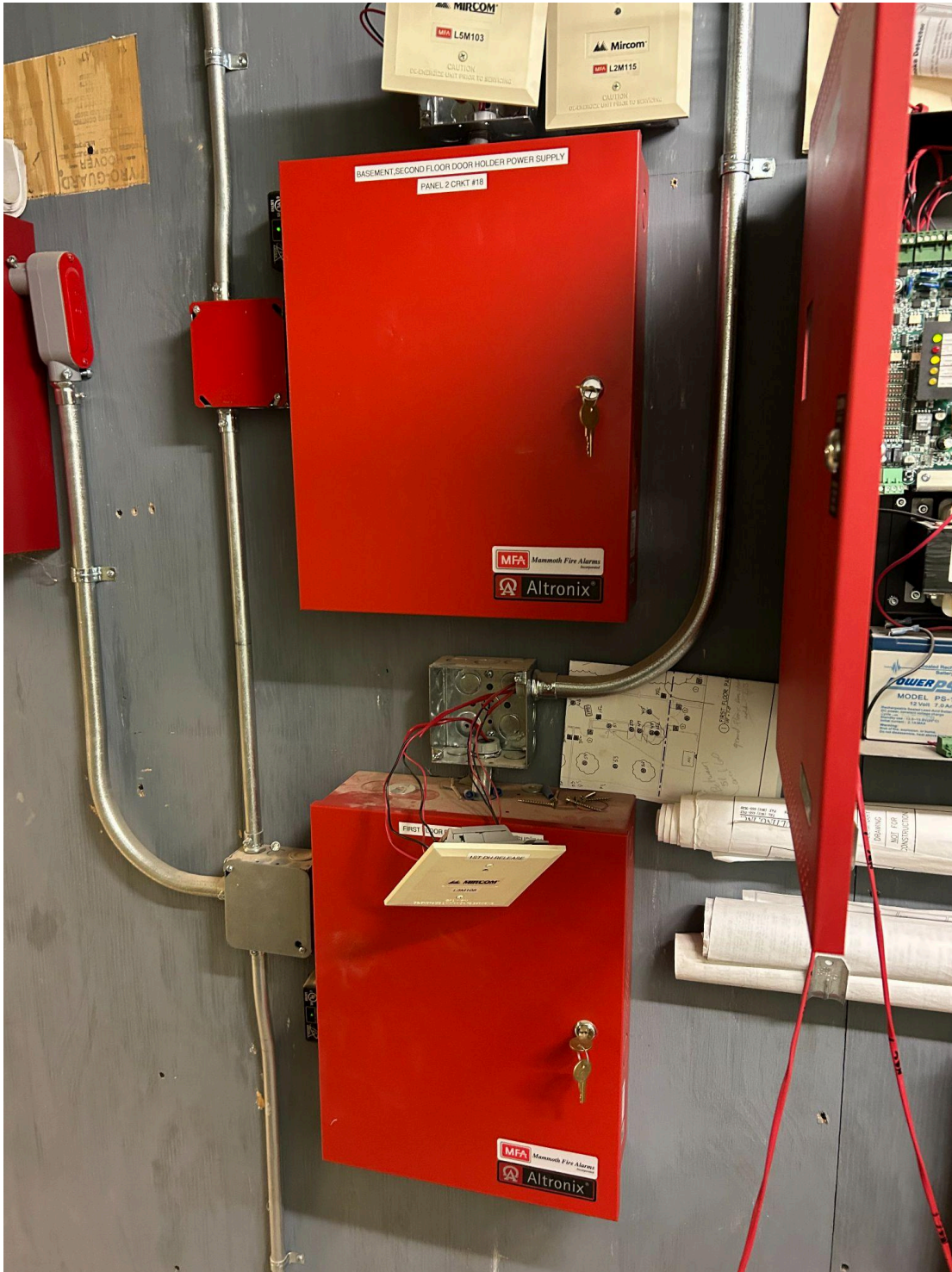
Continued Fire Alarm Subpanels
